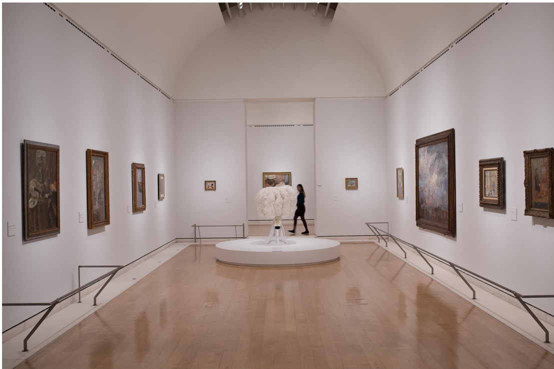
Sackler display gallery, the supply outlets are located at the base of the vaulted ceiling. Air is extracted at the skirting.
